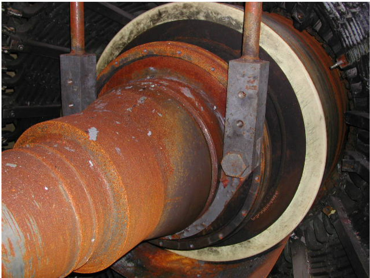
Figure 1: Exciter end of the generator rotor.
