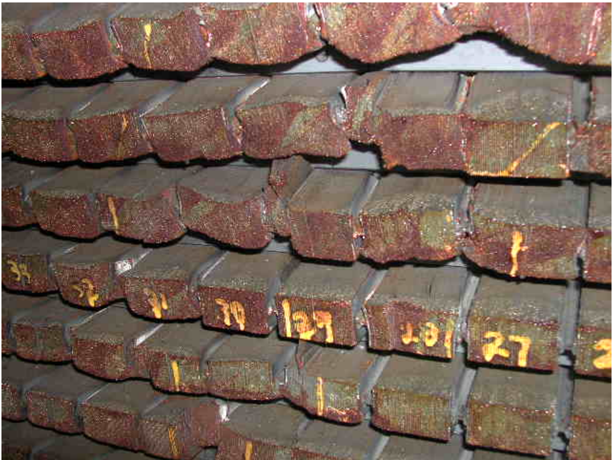
Figure 3: Stator core laminations were displaced due to heat and mechanical pressure over the length of the slot.
