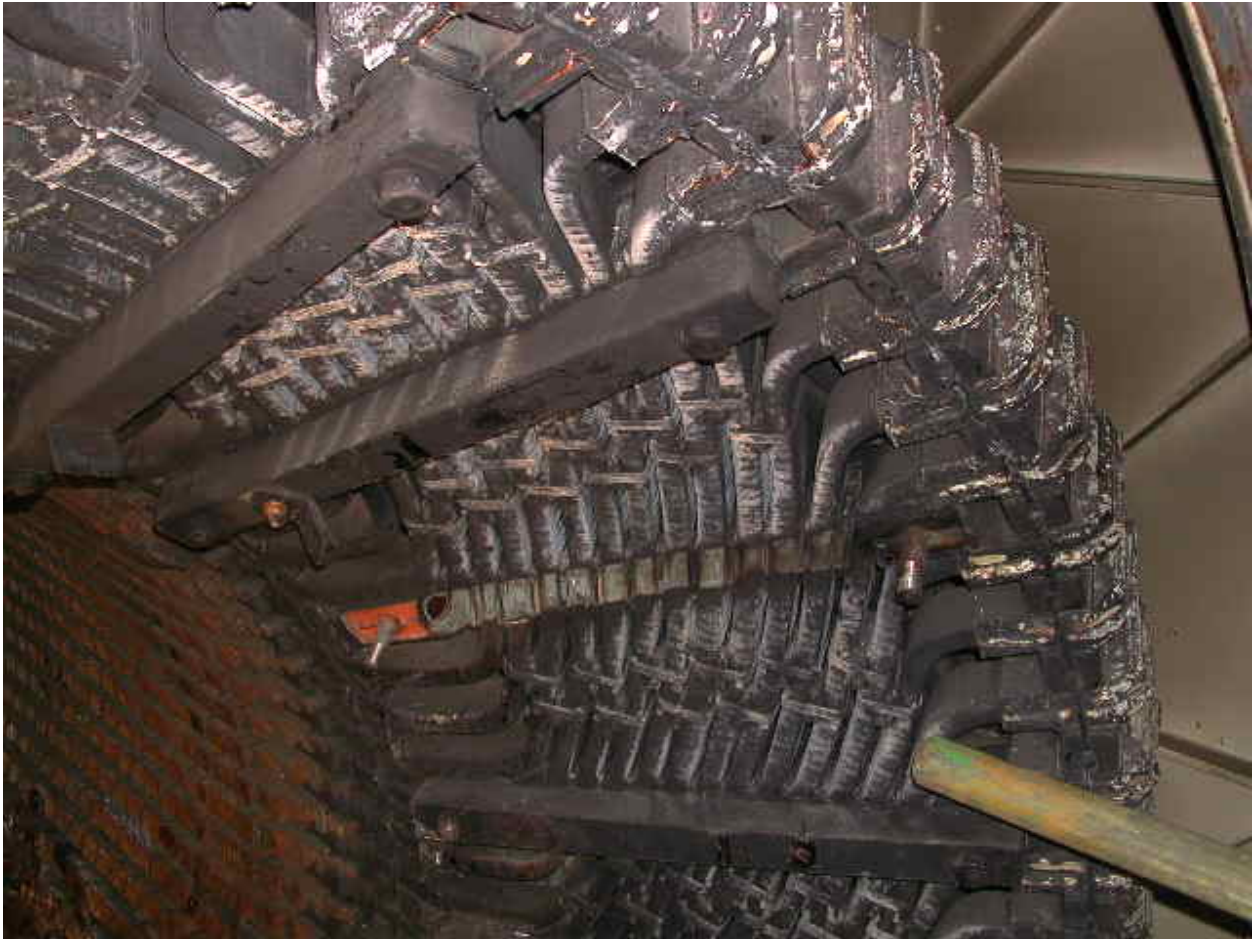
Figure 4: Soot covered exciter end of the generator stator winding is shown above. Notice the heat damage to the insulating clip caps at the ends of the bars.
